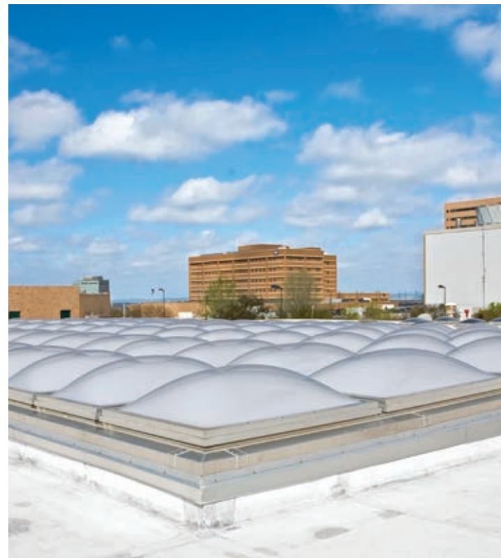
Cluster System, Medical Office Building, San Antonio, TX
