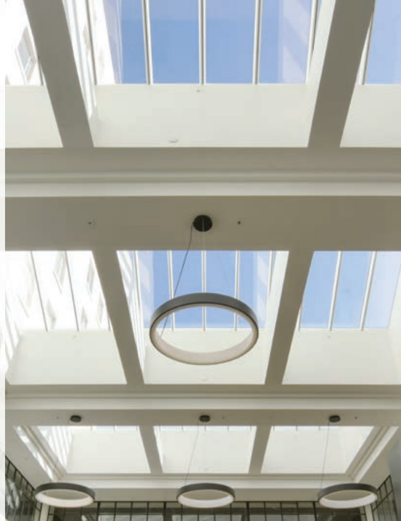
VMS Ridgelight, The Leamington Hotel, Oakland, CA
